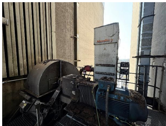
Motor elevator omloop
