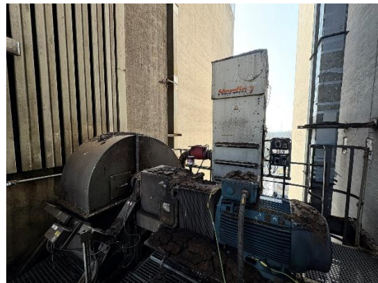
Motor elevator omloop
