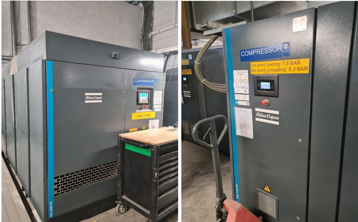
Figuur 14: Compressoren Soliver
