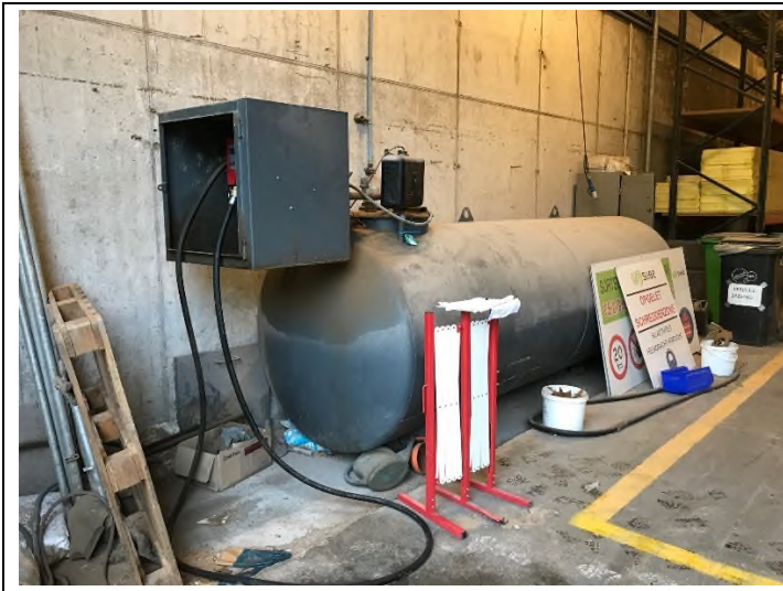
Tank T3 (peilbuis P4/boring B5003)
